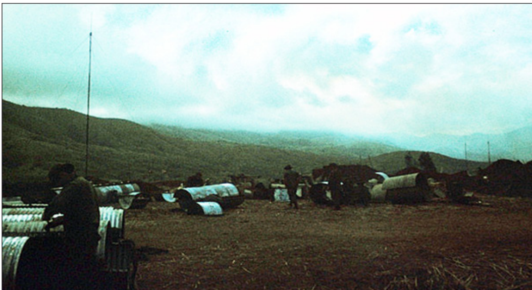
The bridge platoon along with the 2nd platoon began putting the culvert together for placement.
