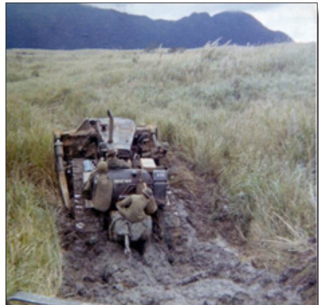
A/7 Engr D7E clearing a path through a low-lying area in the Punchbowl between the Rockpile and Khe Sanh.
